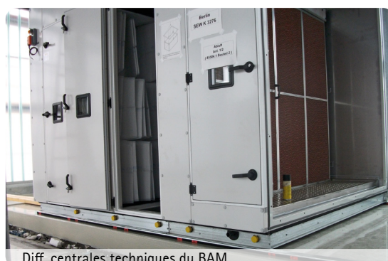
Diff. centrales techniques du BAM
